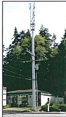
Unacceptable Structure-Mounted Macro Example
