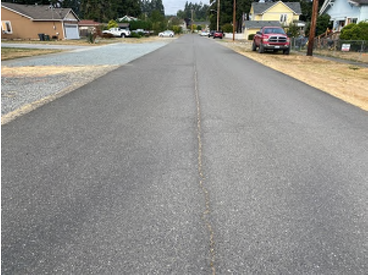
Figure 15. Longitudinal Non-Wheelpath Cracking along Bridge Street
