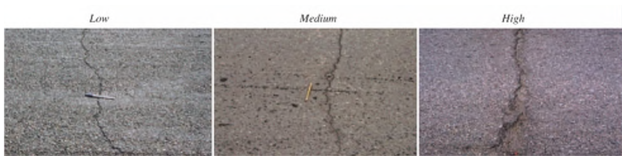
Figure 17. Transverse Cracking Severities
