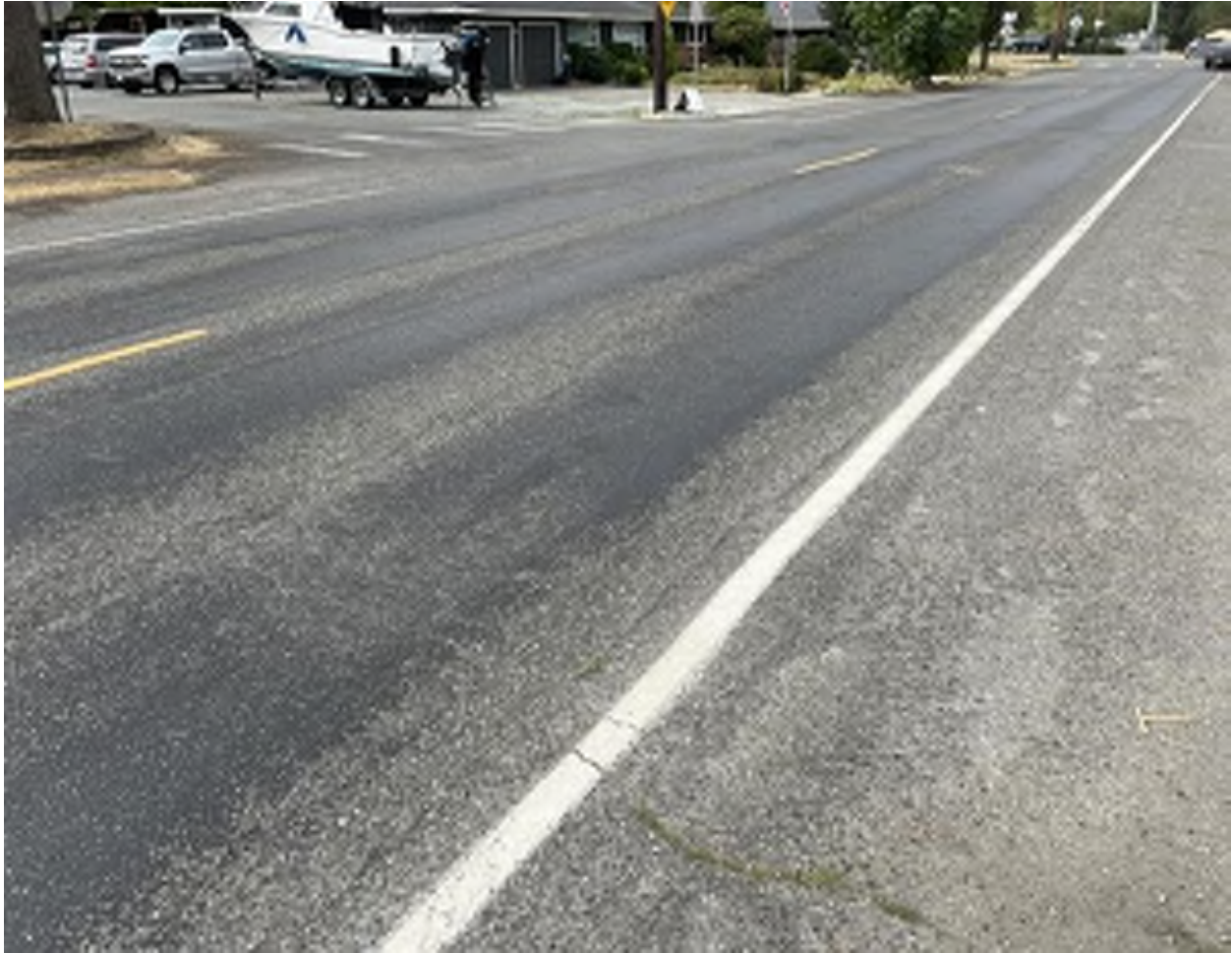
Figure 6. Rutting on Kansas Street
