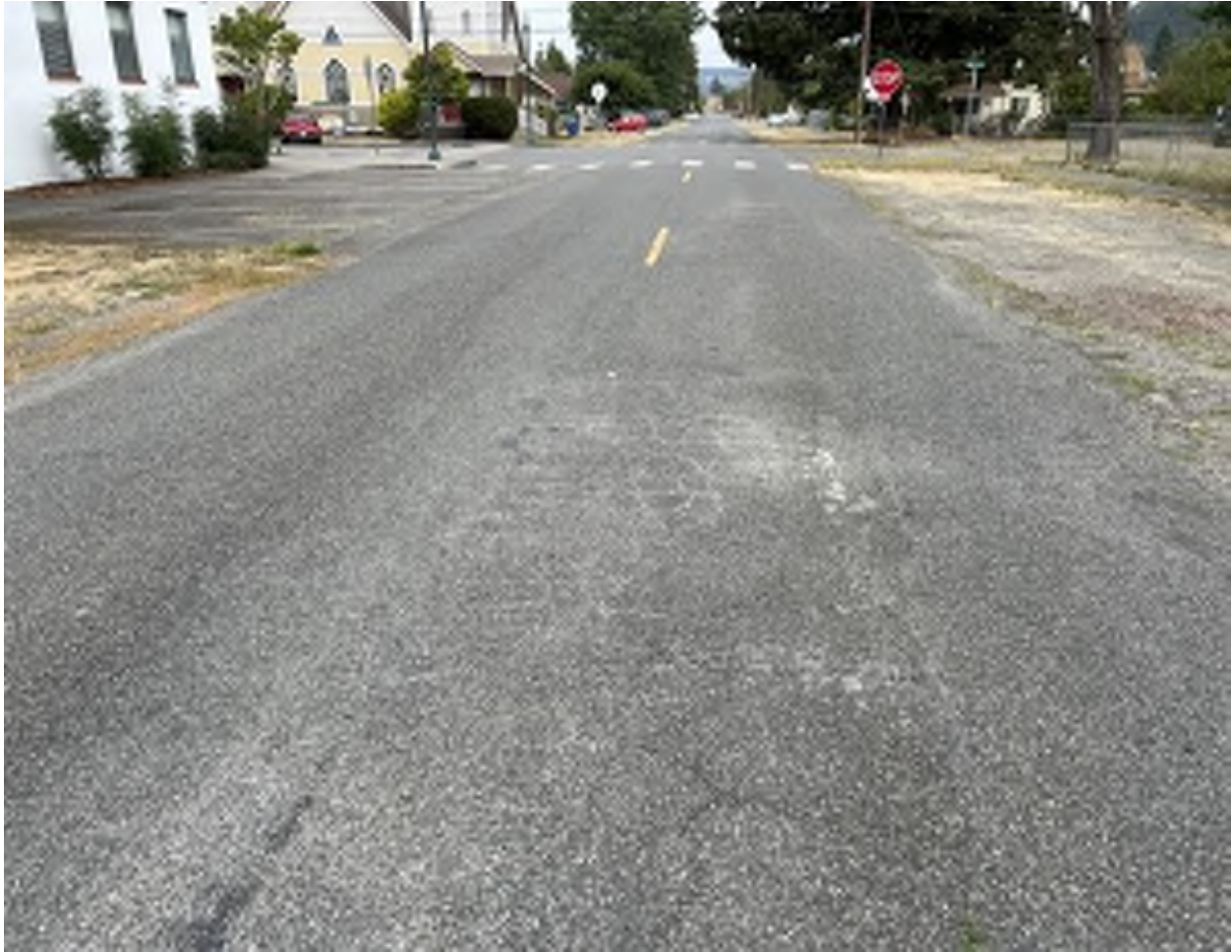
Figure 9. Alligator Cracking on Varner Avenue
