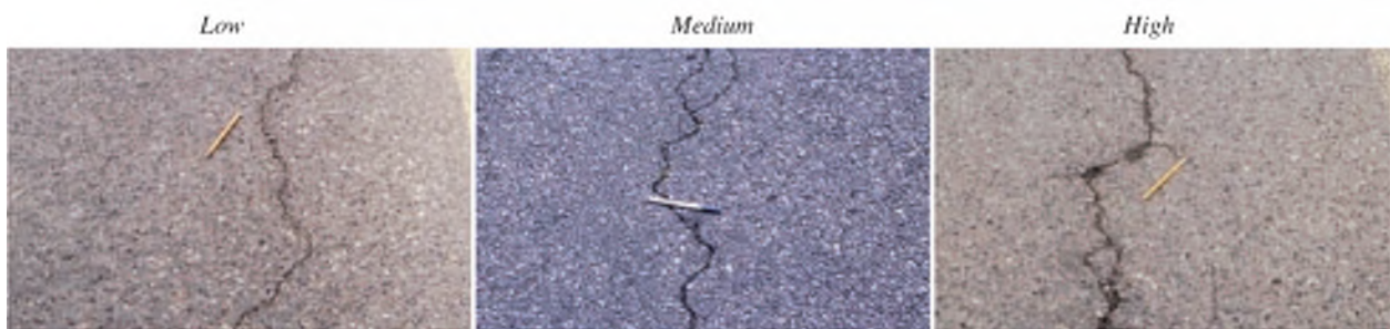
Figure 11. Longitudinal Wheelpath Cracking Severities
