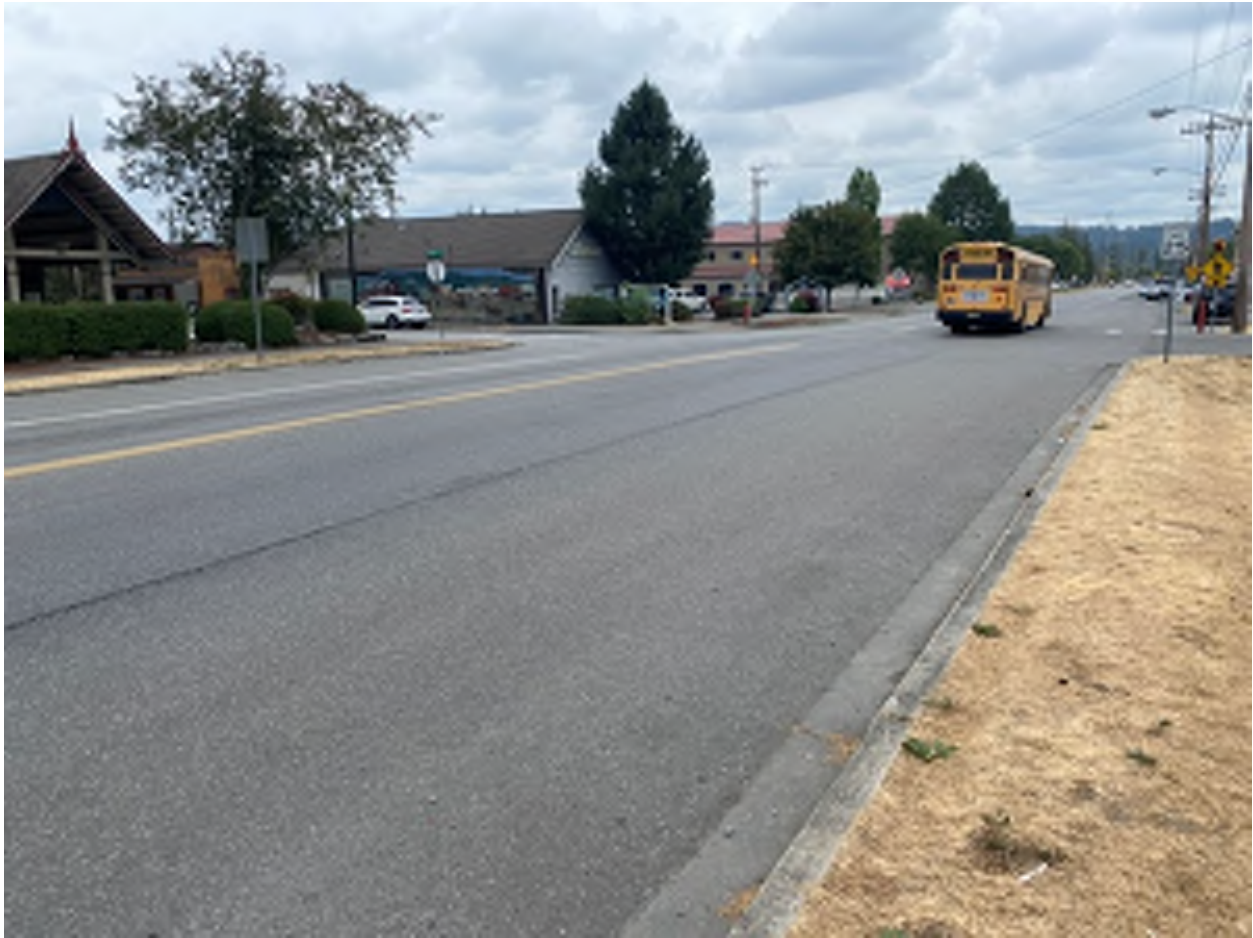
Figure 12. Longitudinal Wheelpath Crack along Calistoga Street
