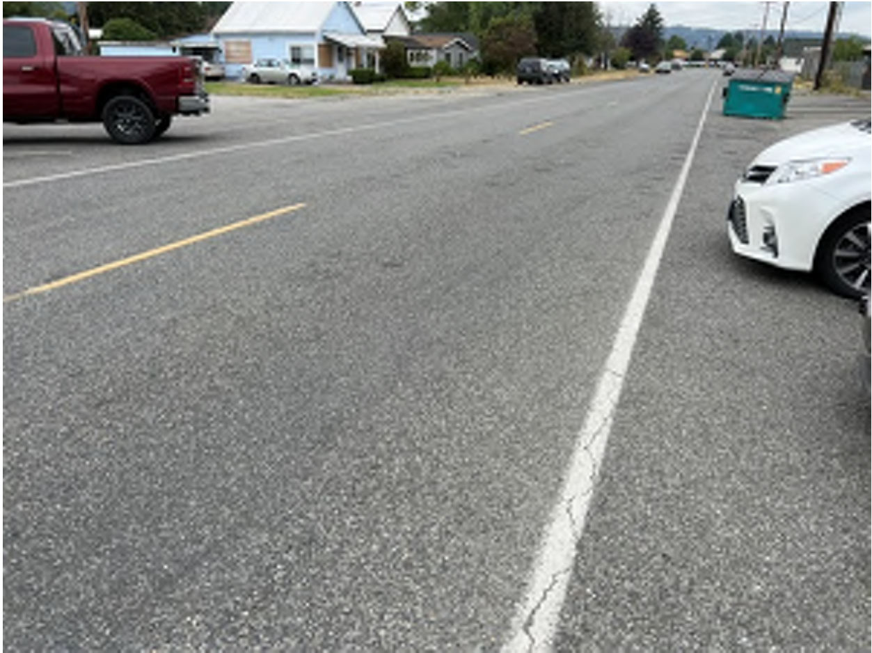
Figure 21. Raveling and Aging along Corrin Avenue
