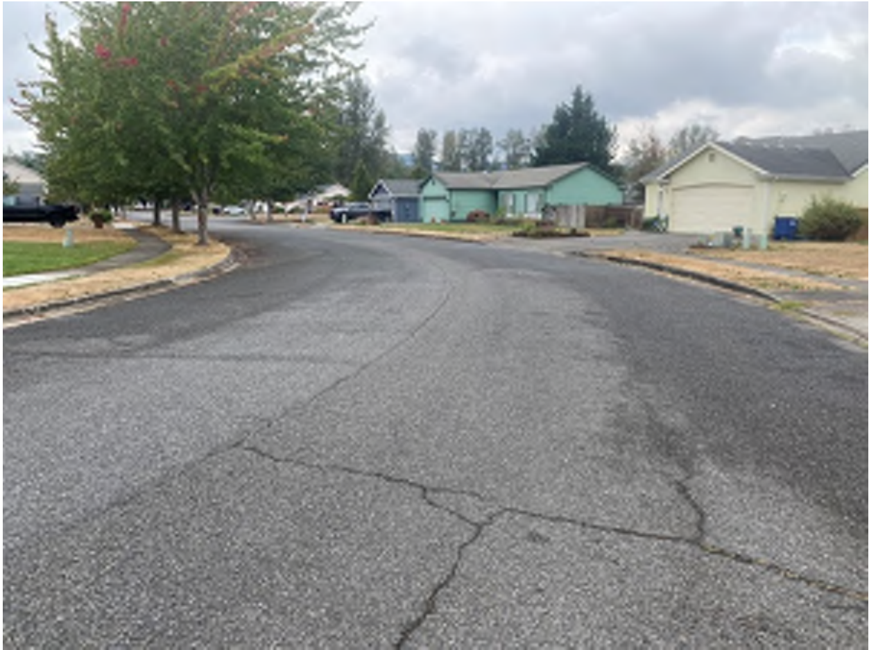
Figure 18. Transverse Cracks on Belfair Avenue
