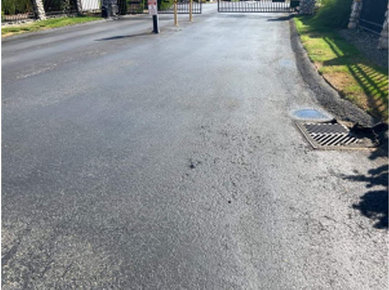
Figure 24. Flushing and Bleeding on Park Place
