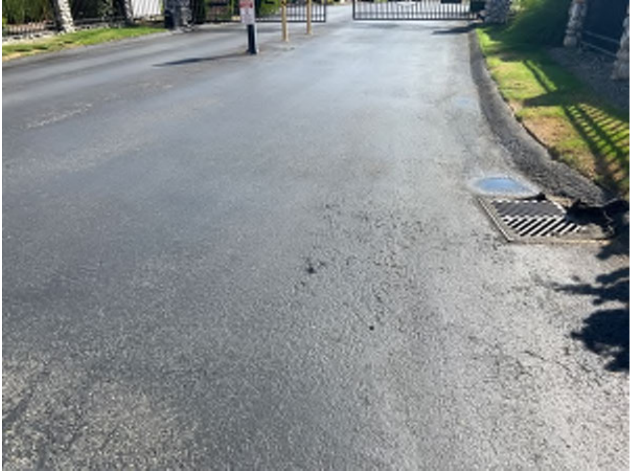
Figure 24. Flushing and Bleeding on Park Place
