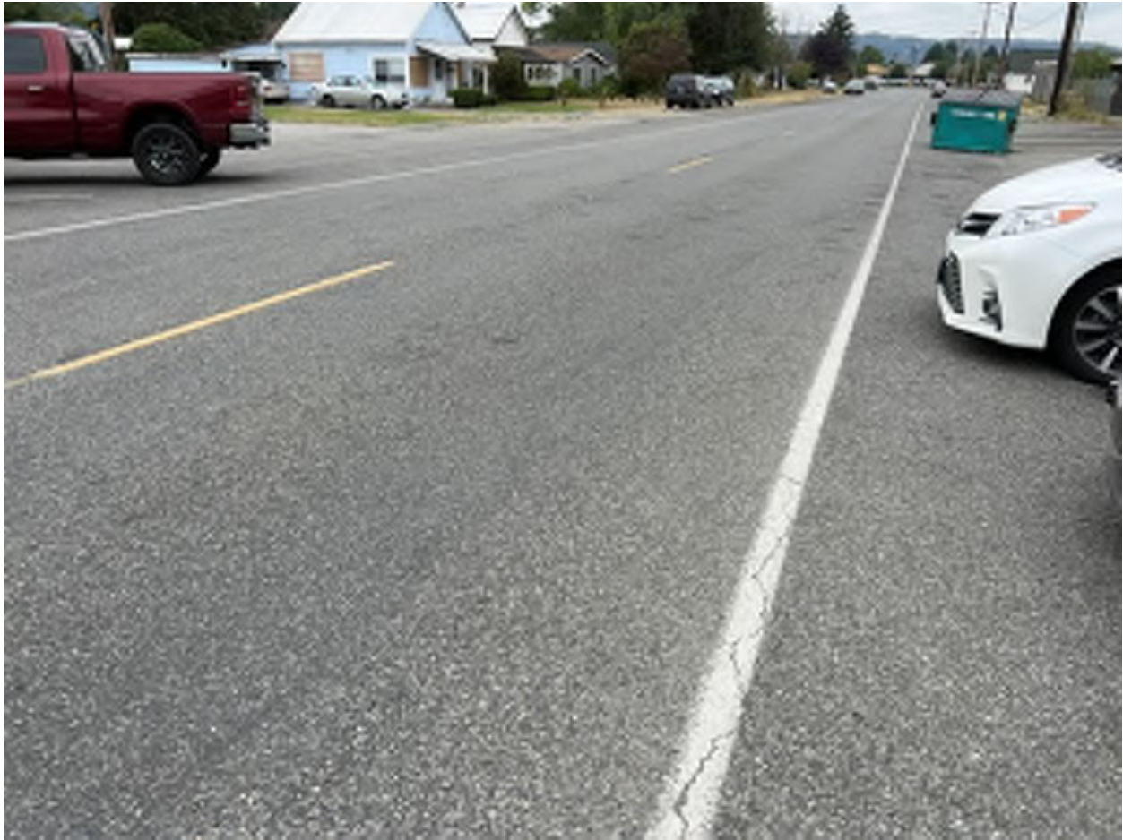
Figure 21. Raveling and Aging along Corrin Avenue
