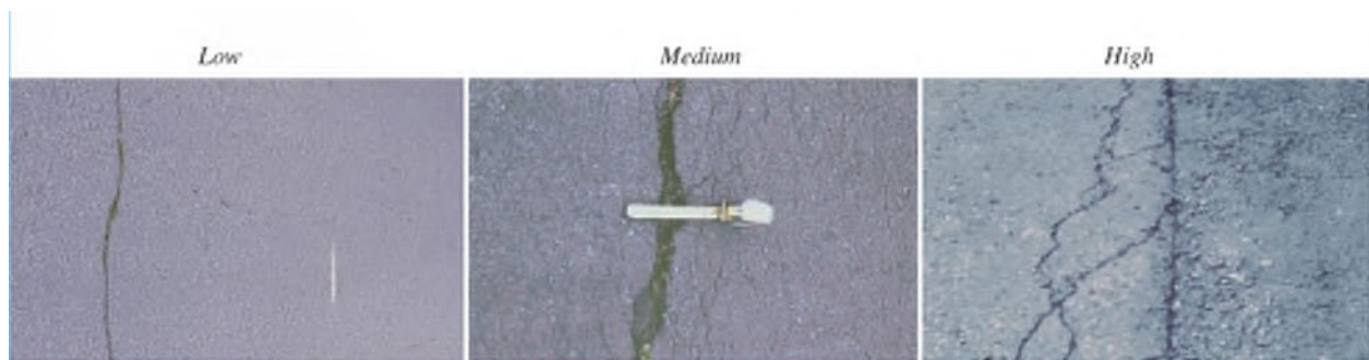
Figure 14. Longitudinal Non-Wheelpath Cracking Severities
