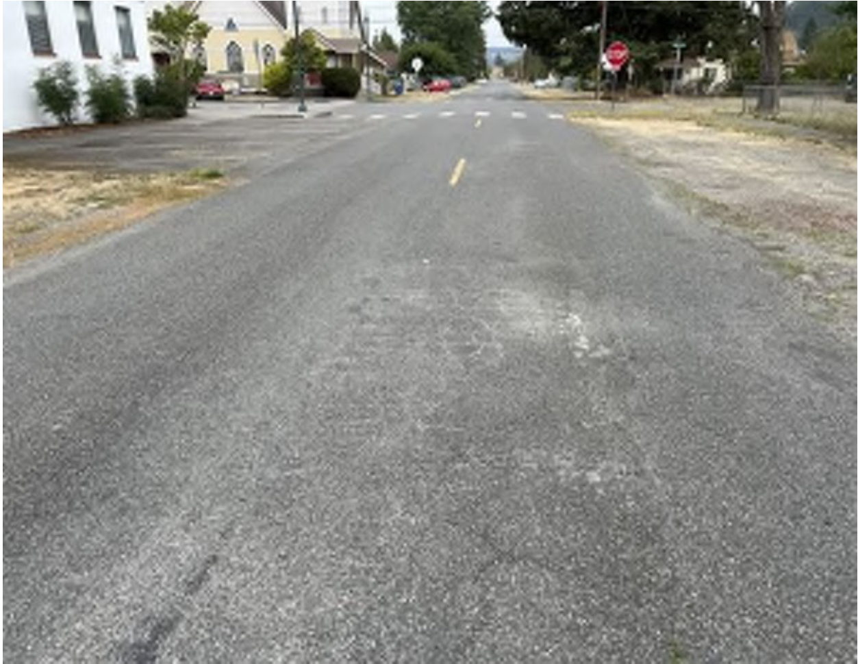
Figure 9. Alligator Cracking on Varner Avenue
