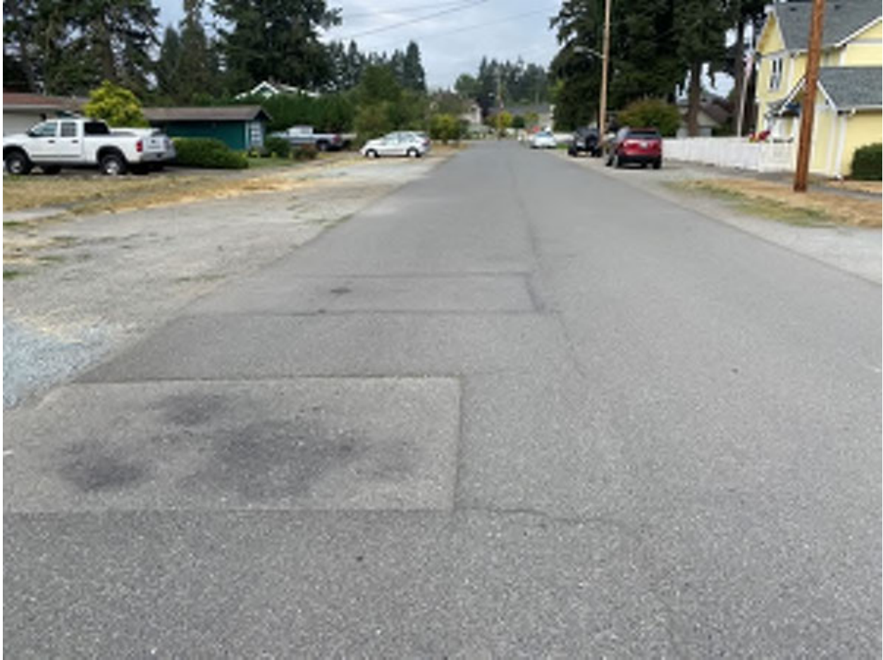
Figure 27. Patching on Bridge Street
