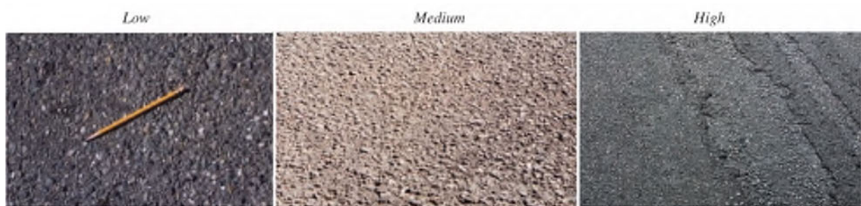
Figure 20. Raveling and Aging Severities
