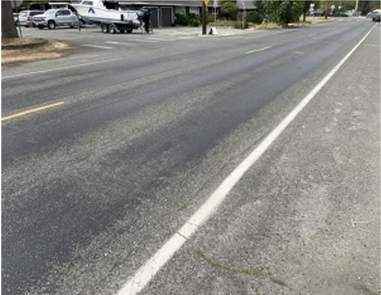
Figure 6. Rutting on Kansas Street
