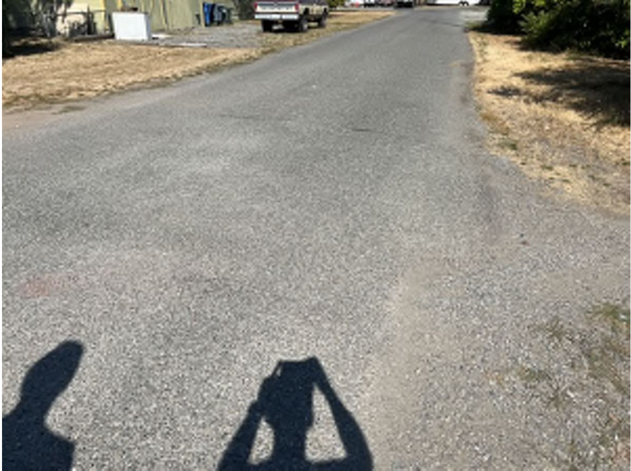
Figure 31. Edge Raveling on Olive Street
