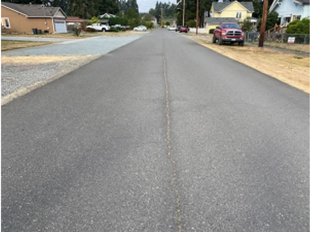
Figure 15. Longitudinal Non-Wheelpath Cracking along Bridge Street
