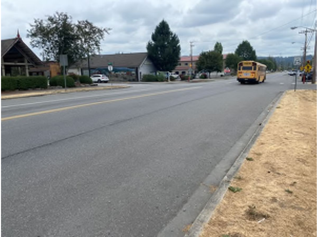
Figure 12. Longitudinal Wheelpath Crack along Calistoga Street
