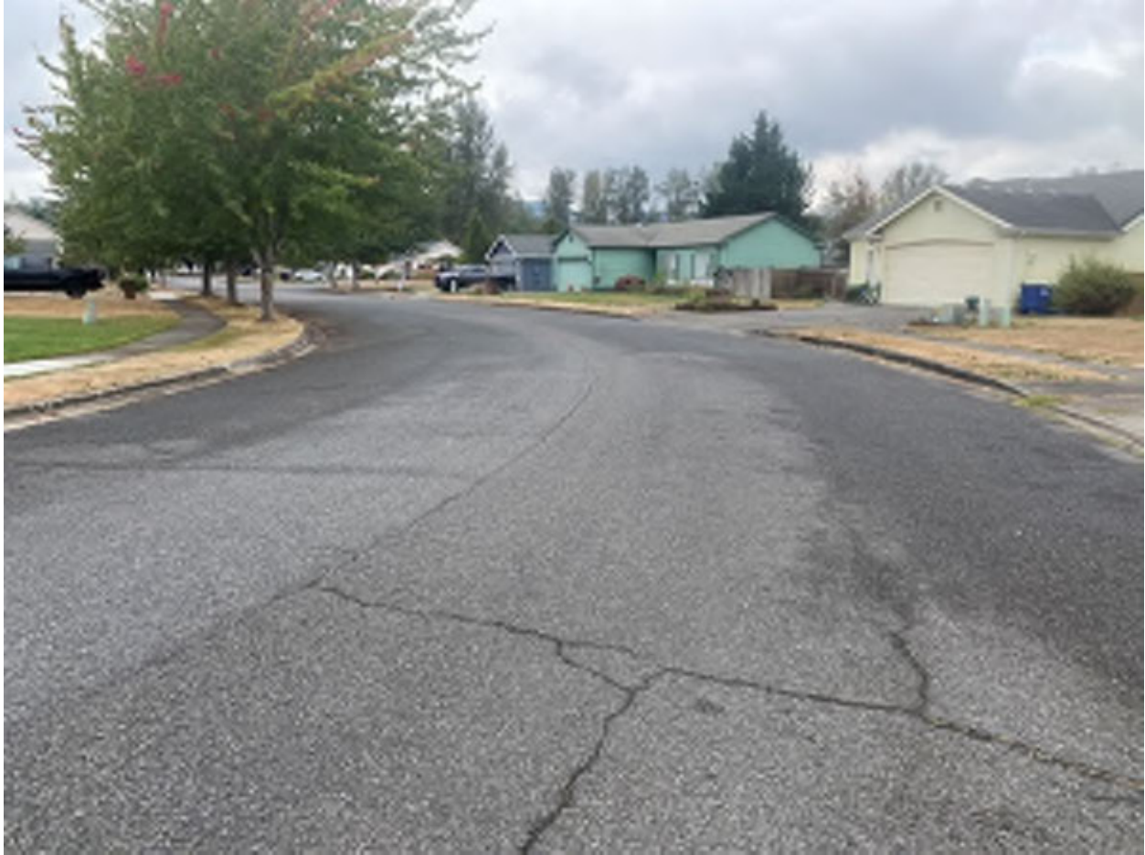
Figure 18. Transverse Cracks on Belfair Avenue
