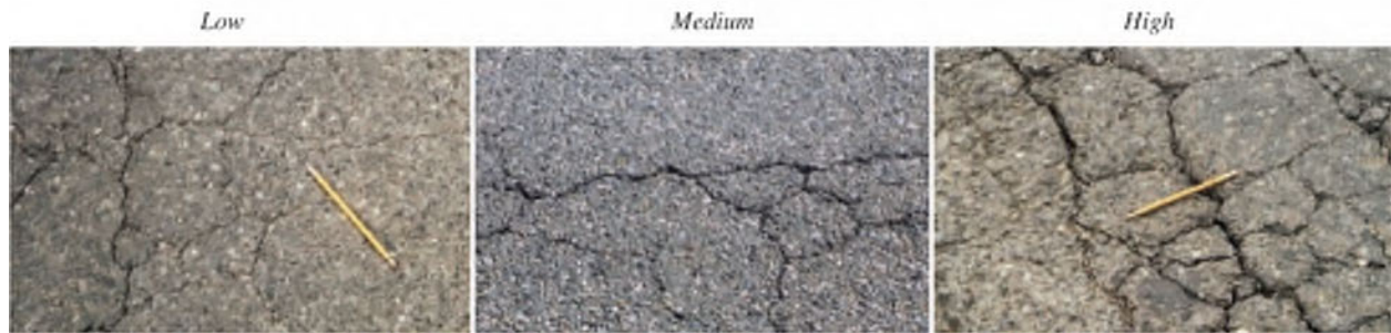
Figure 8. Alligator Cracking Severities
