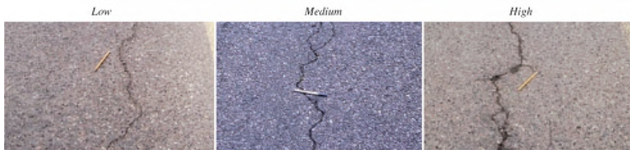
Figure 11. Longitudinal Wheelpath Cracking Severities
