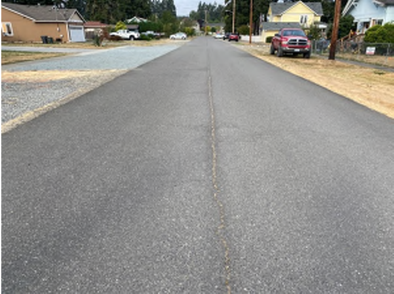
Figure 15. Longitudinal Non-Wheelpath Cracking along Bridge Street
