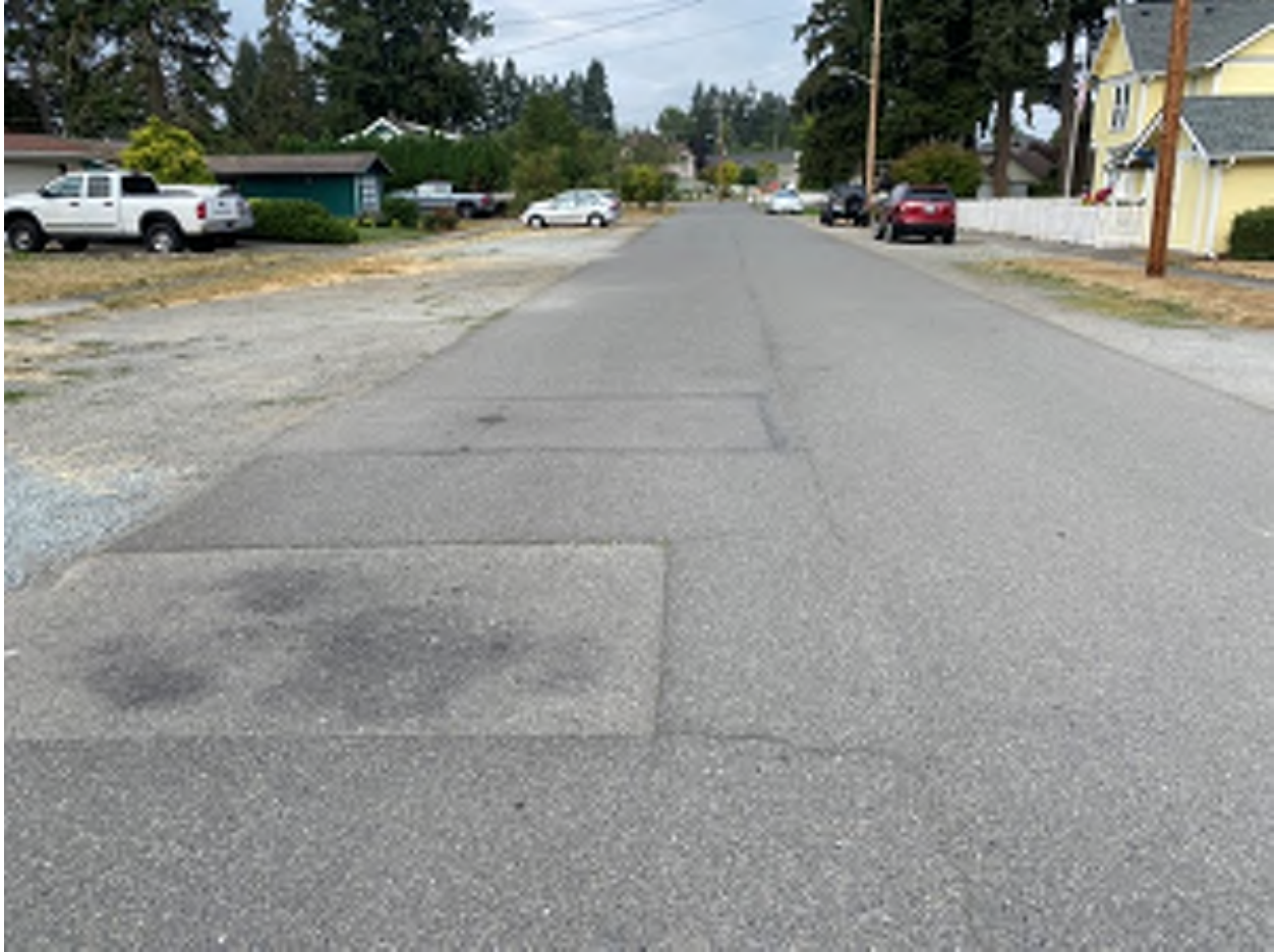
Figure 27. Patching on Bridge Street
