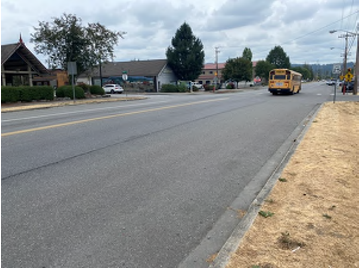
Figure 12. Longitudinal Wheelpath Crack along Calistoga Street
