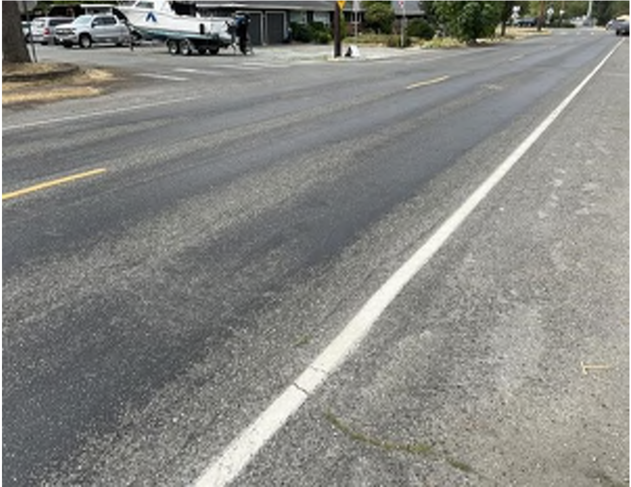
Figure 6. Rutting on Kansas Street
