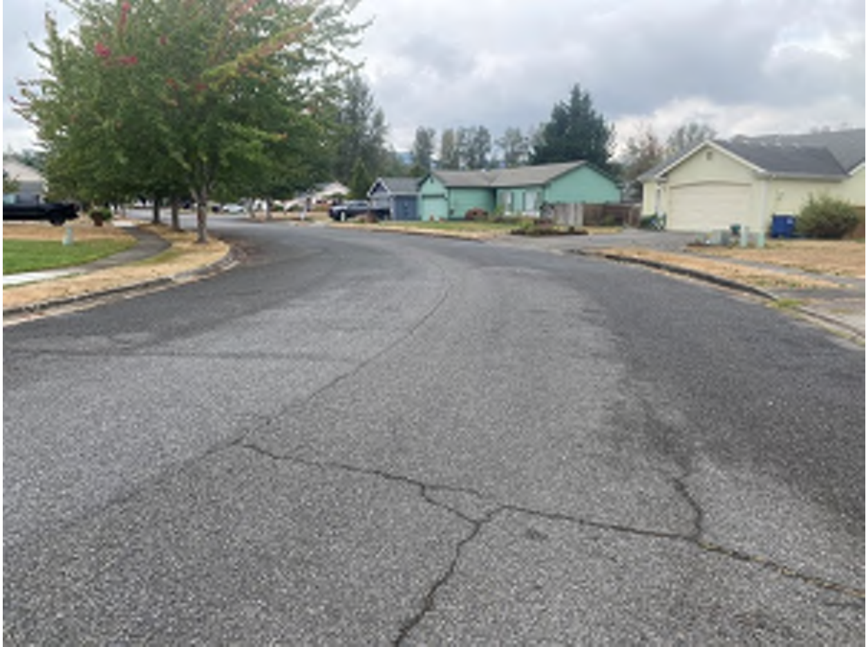
Figure 18. Transverse Cracks on Belfair Avenue
