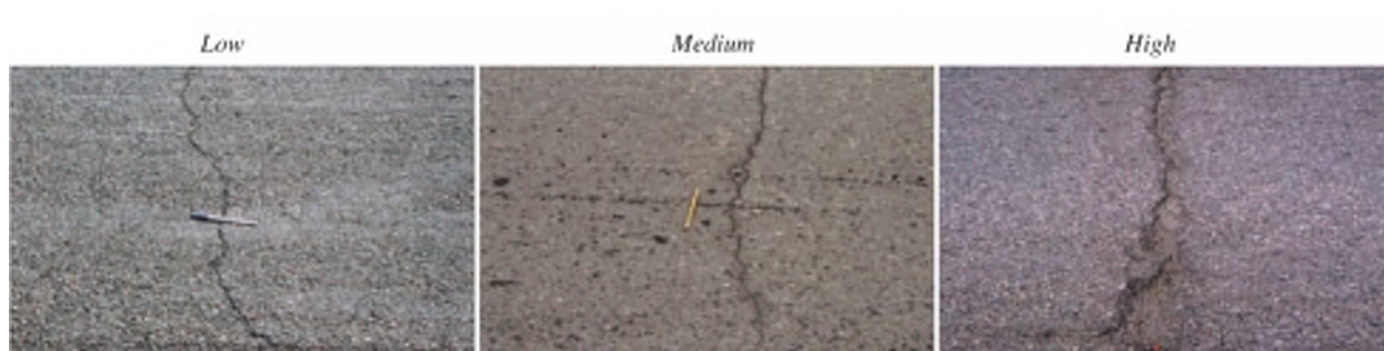
Figure 17. Transverse Cracking Severities
