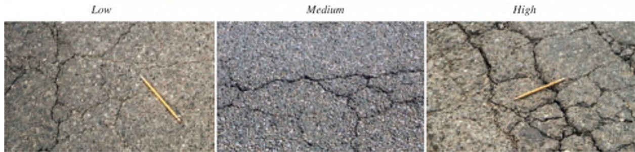
Figure 8. Alligator Cracking Severities
