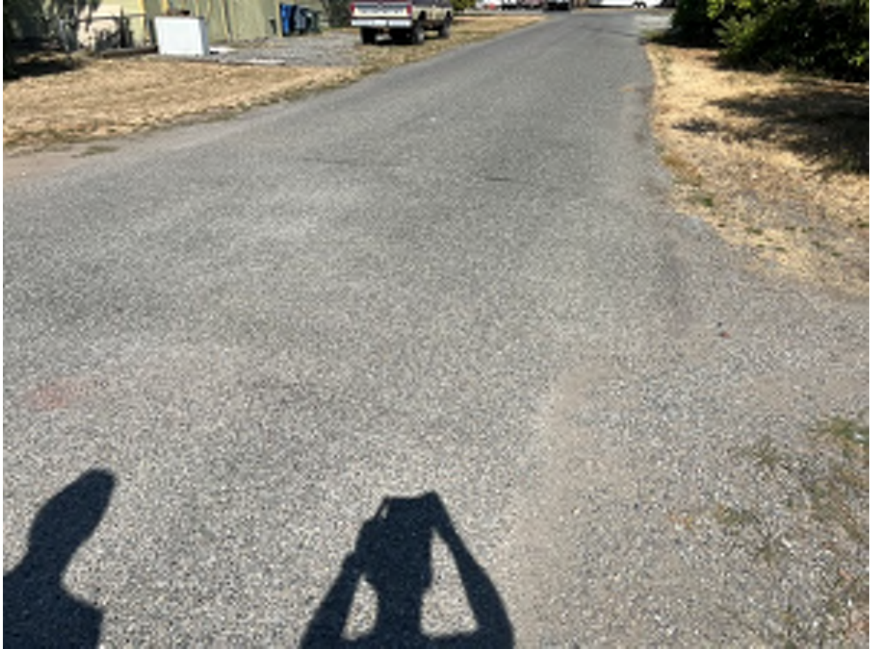
Figure 31. Edge Raveling on Olive Street
