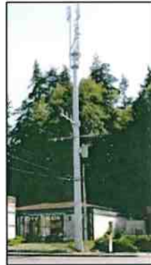
Unacceptable Structure-Mounted Macro Example
