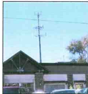
Unacceptable Monopole Macro Example
