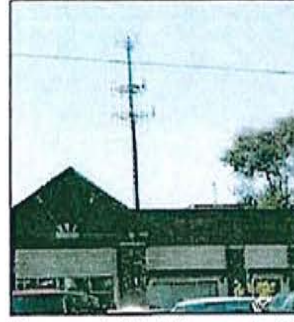
Unacceptable Monopole Macro Example
